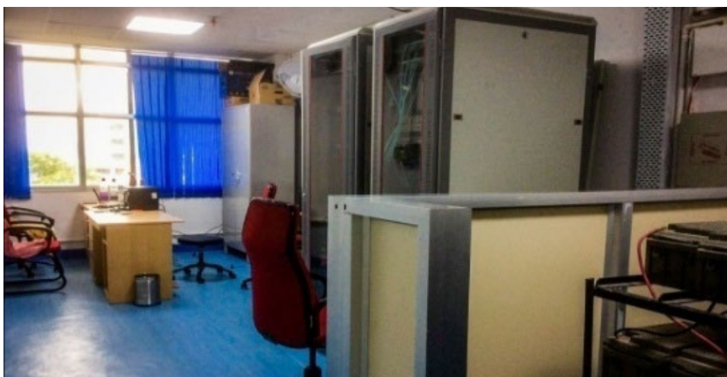
Salt Lake Campus Server Room
