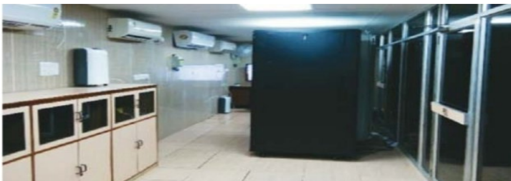
Jadavpur Campus Server Room
